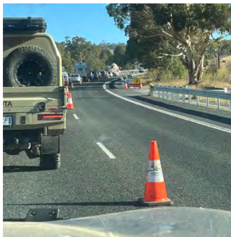
Works being undertaken to repair a defect at the start of the new southbound overtaking lane. Photo: Michael Evans
