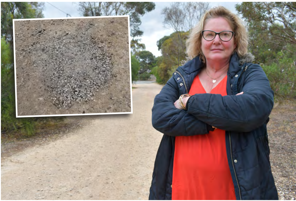
Willyaroo resident Mandy Melville has grown increasingly frustrated by the reoccurring potholes on Blacker Road. INSET: The reoccurring holes are currently being filled in by the neighbours. Photos: Giorgina McKay
